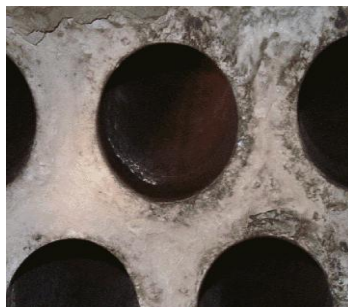
Clean boiler tubes provide optimal heat transfer.
