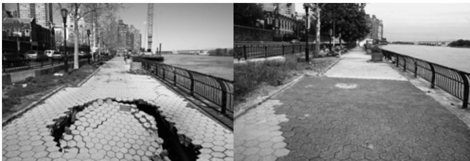
Gaping holes in the East 70s of the Esplanade have been repaired thanks to funding secured by elected officials. Left: As seen spring 2011. Right: As seen summer 2011. Photos by Anton Brookes, www.mockturtlemoon.com
