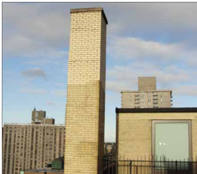
When switching to natural gas, a chimney liner is required for masonry chimneys. A chimney inspection will determine if a liner is necessary. Most buildings with pre-1950 masonry chimneys, as shown in the picture above, will need to install a chimney liner.
